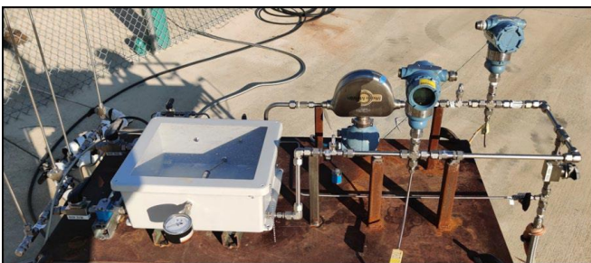
Figure 2: Example of H 2 Blended NG Flow Rig
