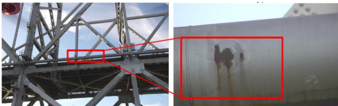
Figure 4: sUAS corrosion detection location results, GPS specific identification, pipe bridge 750 feet above a navigable waterway
