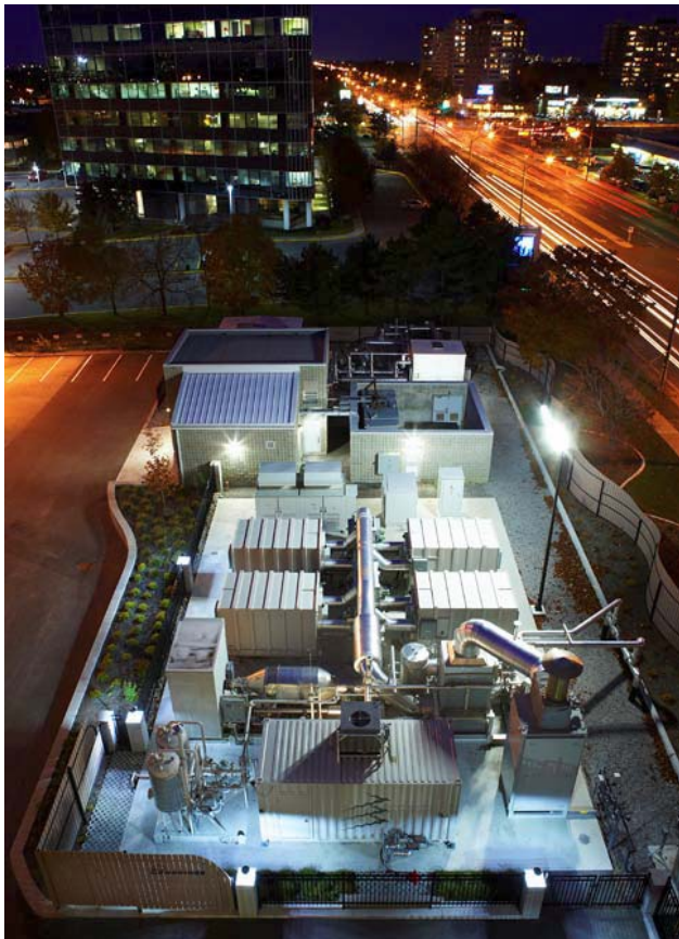
Figure 2: 2.2MW Ultra-Clean Hybrid Power Generation Facility Located at an Existing Urban Gate Station.
