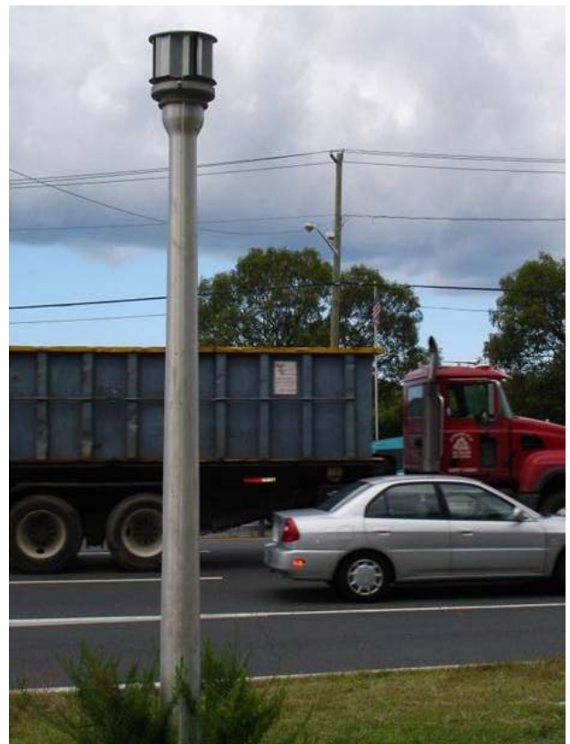
Figure 1: Urban-Style Cased Pipe Casing Vent
