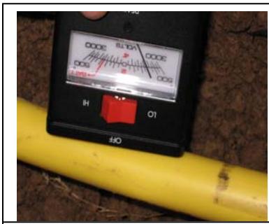
Static Voltage Reading on Exposed PE
