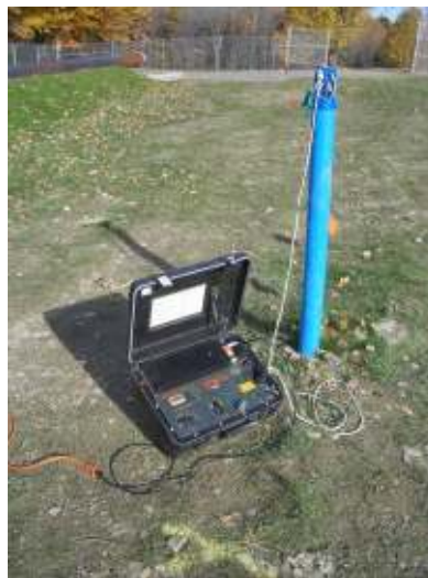
PCM Tx Connected to a Test Station
