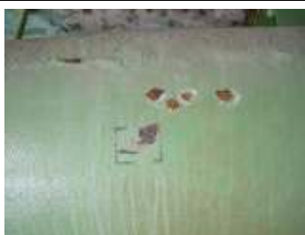
Minor Corrosion Revealed
