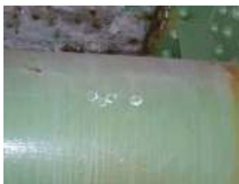
Areas of Predicted Corrosion
