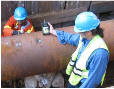
Ultrasonic Thickness Gage Verification
