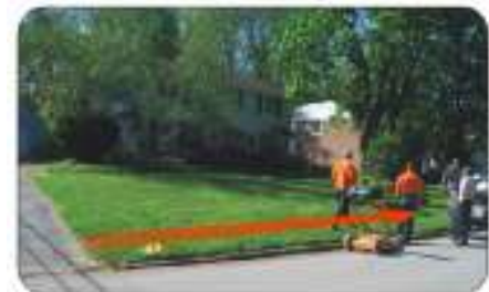
Harris System in Live PECO field tests
