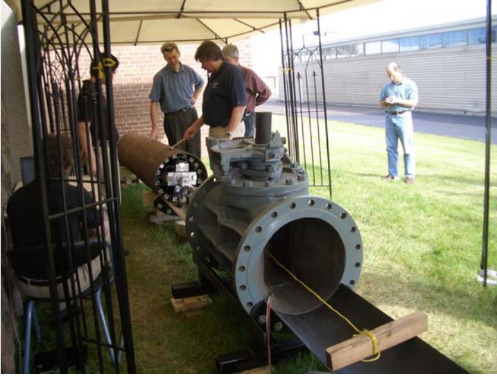
Another view of the technology observed by (l to r) Bill O'Brien, Invodane (with back to camera); Roderick Lee, Invodane; Poul Laursen, Invodane; George Ragula, PSE&G [NYSEARCH Chairman]; Joe Vitelli, KeySpan; and Joe Mallia, Rochester Gas & Electric.
